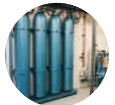
High Pressure Air Storage
