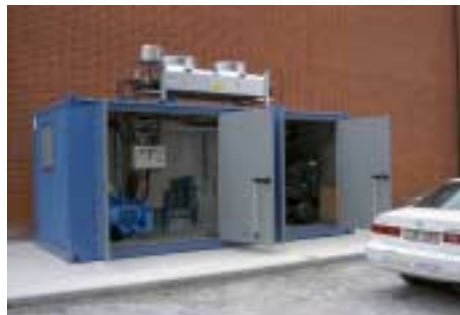
High Pressure compressor system for medical breathing air for AGA Linde Healthcare, Rotebro.
