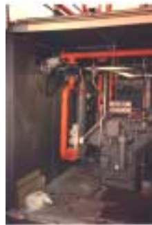
Inside of Natural gas compressor plant.
